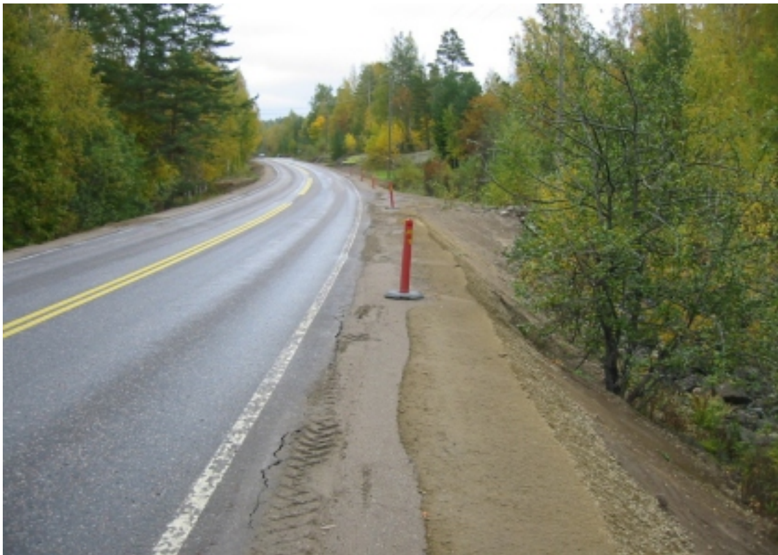
Figure 14. Pilot 2003. Safety lane in connection to the main road Kt 322, during construction in 2003.
