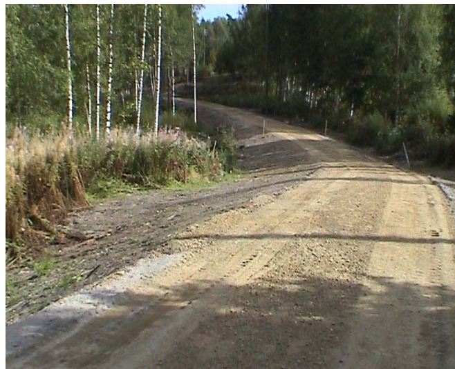
Figure 7: A section of the new light traffic lane, pending final covering course and finish of the slopes. Luopioinen, summer 2003.
