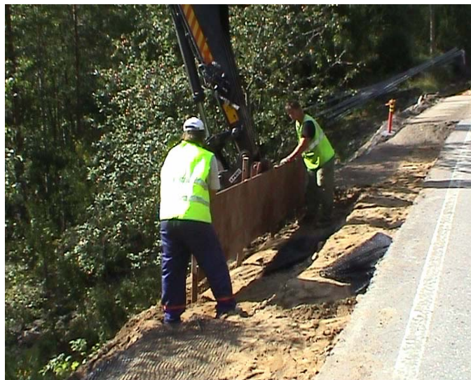
Figure 10: Supporting plate used for the construction of the safety lane at a steep site. Luopioinen, early autumn 2003.
