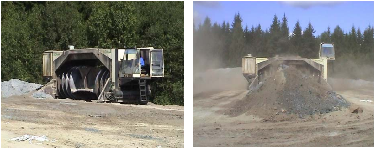
Figure 4: Stack mixing for Pilot 2003 Fibre-ash. Left: the stack mixer. Right: the stack mixer working with a stack of fly ash and fibre-clay. Because of dusting the mixing site must be chosen carefully and the workers must be equipped with respirators. Luopioinen, summer 2003.
