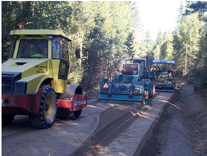
Figure 3: Stabilisation is going on at Pilot 2002 road. In the background the spreading machine, in the middle the milling cutter, and in the front the roller. Luopioinen, summer 2002.
