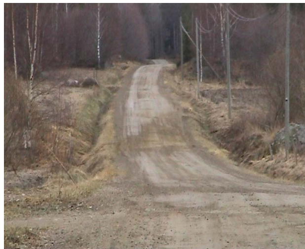
Figure 1: Frost damage of a gravel road. Luopioinen 2002
