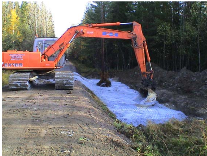
Figure 6: Compaction of fibre-clay going on. The compacted fibre-clay course should act as an impermeable sealing course of the groundwater protection structure. Early autumn 2003, Luopioinen.
