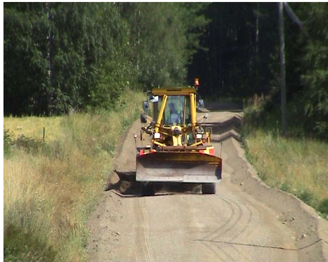
Figure 5: Working of the edge supports is going on for the pilot road. Luopioinen, summer 2003.
