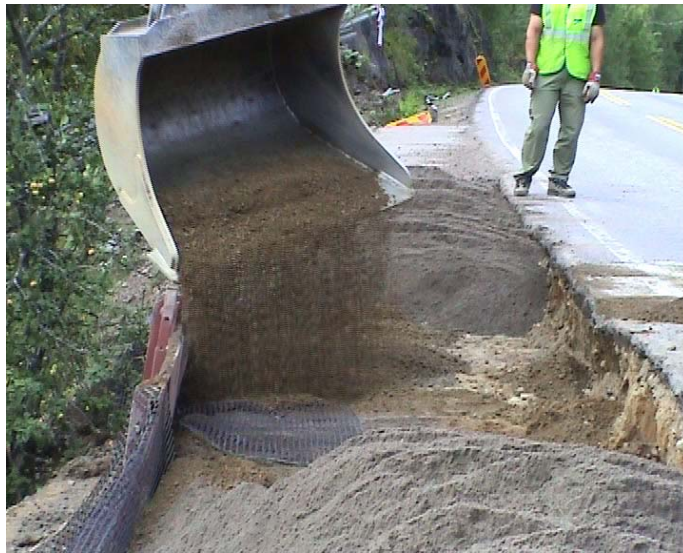
Figure 9: Works going on at the fibre-ash section of the safety lane. Luopioinen, early autumn 2003.
