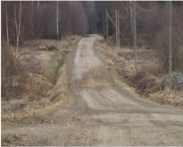
Figure 1: A damaged section of a gravel road in Luopioinen in 2002
