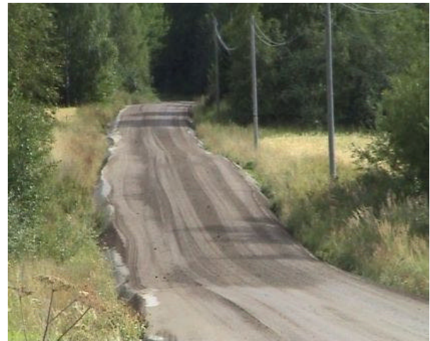
Figure 2: Intermediate level. The gravel road during renovation, before finishing with covering course. Luopioinen Summer 2003, renovation with a fibre-ash structural course.
