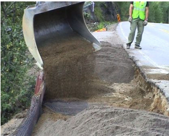
Figure 8: The on-going safety lane construction where the fibre-ash course is bound inside a geonet before compaction and covering course.
