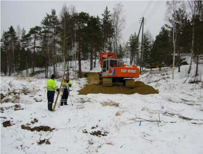
Figure 1: Pre-loading for the light-traffic lane running on a soft peat area. Pilot 2003
