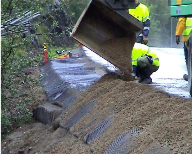
Figure 4: Crushed aggregate to cover the geonet containing the fibre-ash course. The compaction will be made on the crushed aggregate. Pilot 2003
