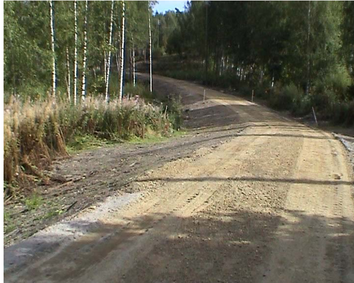
Figure 1: Light-traffic lane in Luopioinen in August 2003. Only the final covering course is missing.
