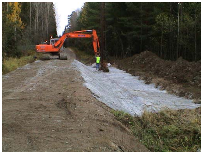
Figure 4: Compaction of fibre-clay for the impermeable sealing course of the groundwater protection structure. Luopioinen 2003.
