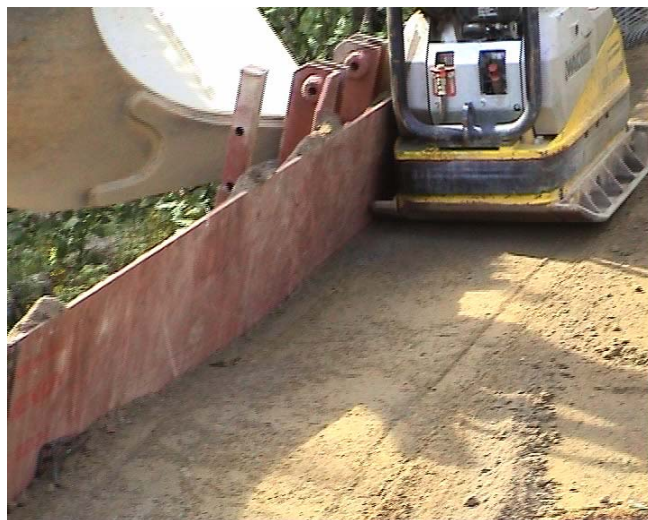
Figure 2: The support plate for the safety lane construction, and compaction on a crushed aggregate course. Luopioinen 2003
