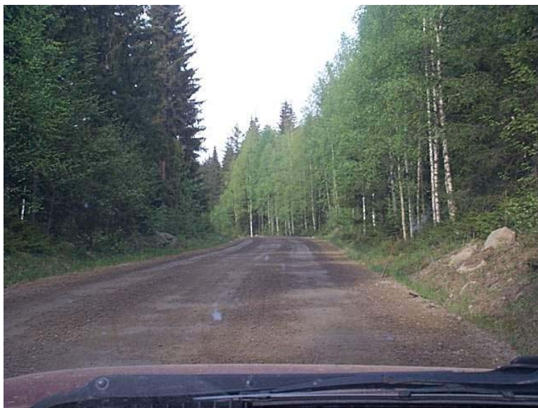
Figure 1: Frost damage of a gravel road section in the spring 2002. Luopioinen
